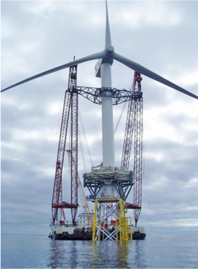
OWEC Jacket Foundation at Beatrice Offshore Wind Project
